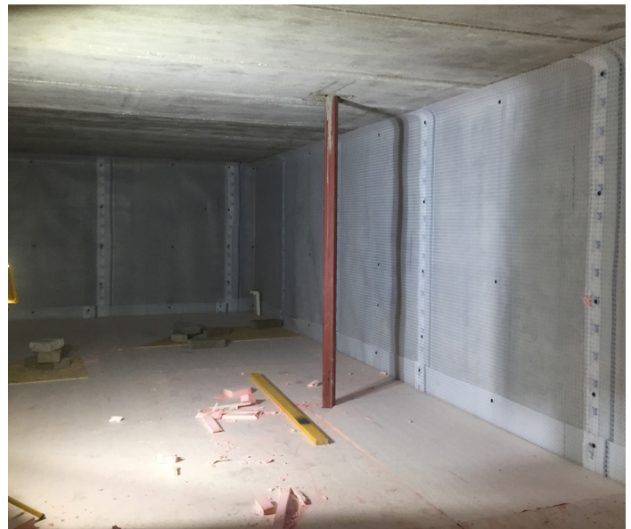
Type C Newton CDM System was installed internally.
