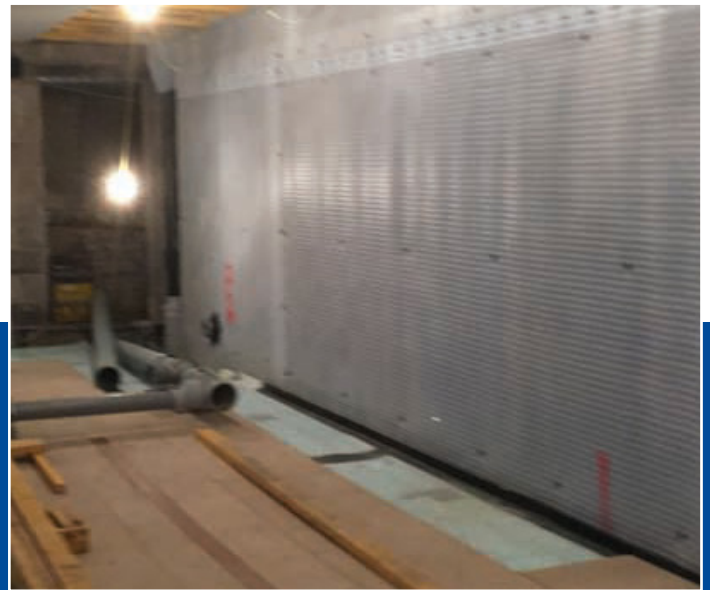
The CDM system uses sump and pump systems to remove water.
