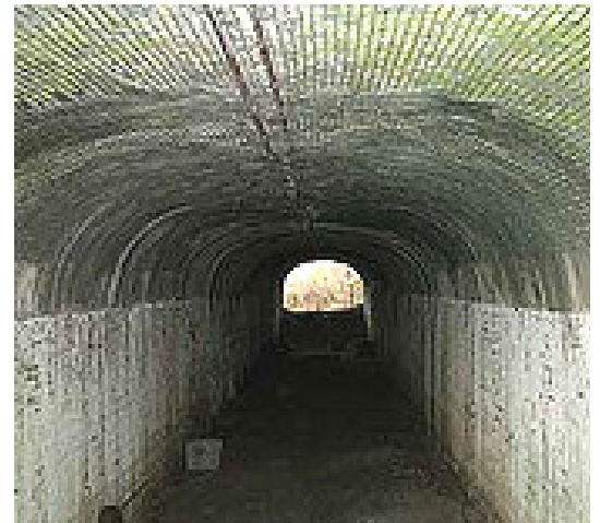
Charmouth Tunnel suffered from severe damp
