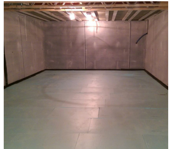
The original concrete structure was leaking.
