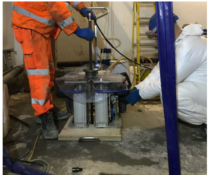
The 320-FP reacted with the ground water to quickly provide a seal.
