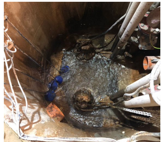
The cracked tank was allowing ingress of groundwater.
