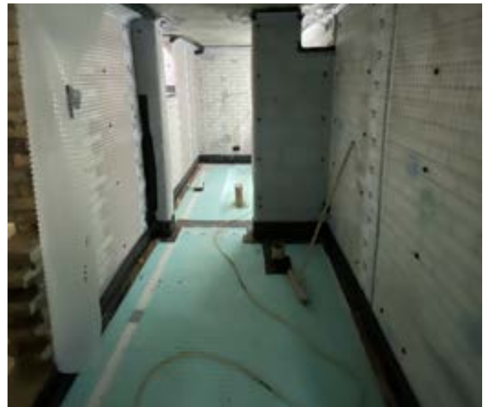
Waterproofing was required to the main body of the house at this level.
